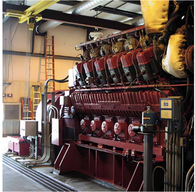
H.W. Hill Landfill Gas Project engine. Source: Republic Services
